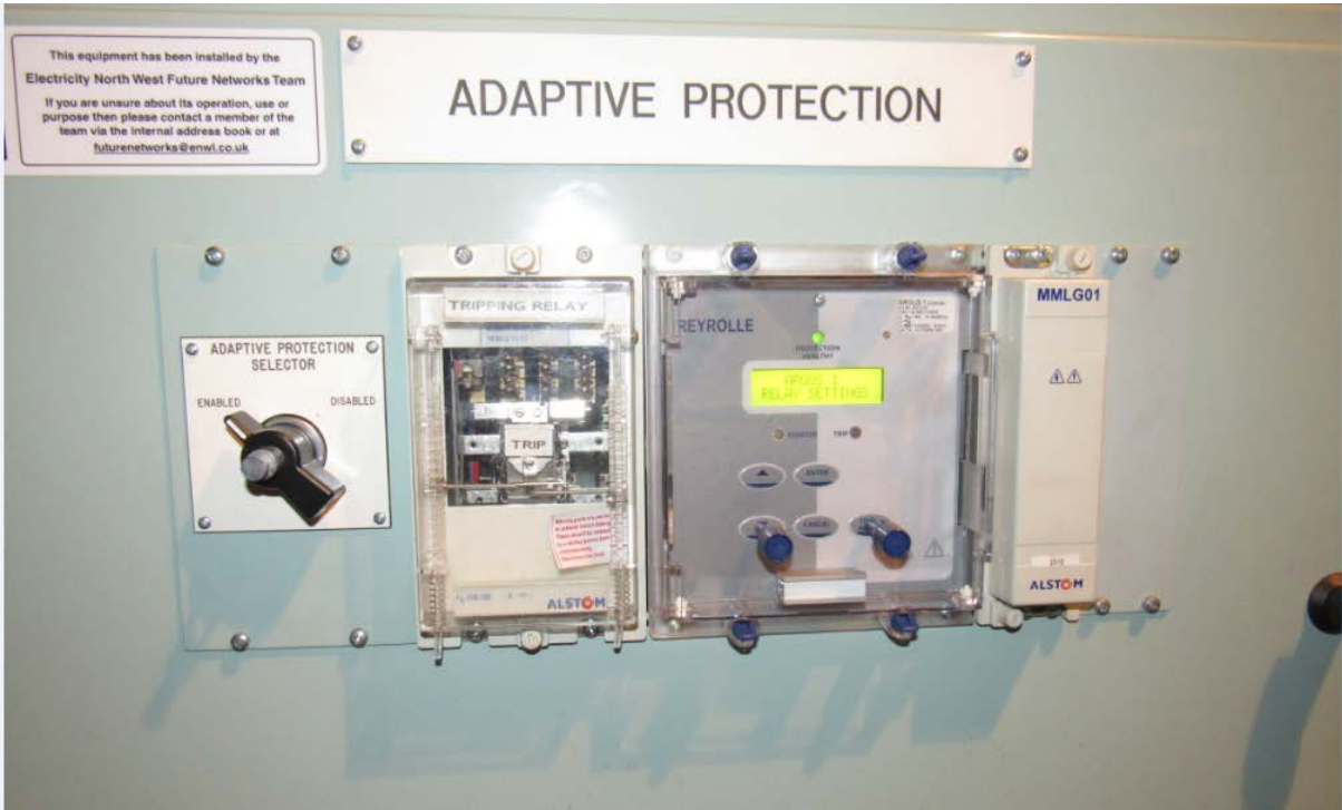
Photograph 2: Adaptive Protection and tripping relays
