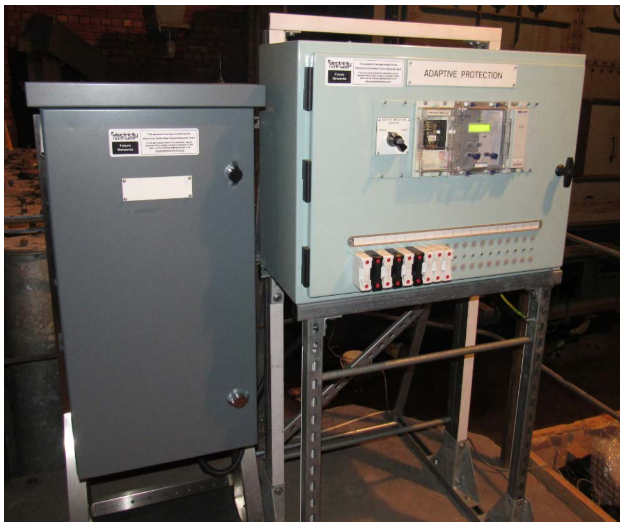
Photograph 1: RTU and Adaptive Protection panel
