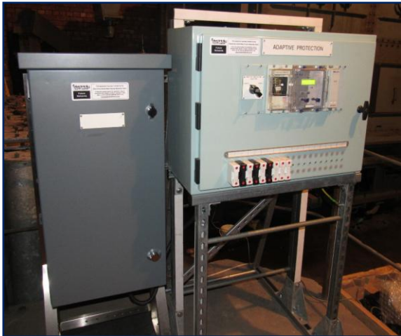
Figure 3.17: Remote terminal unit and adaptive protection panel
