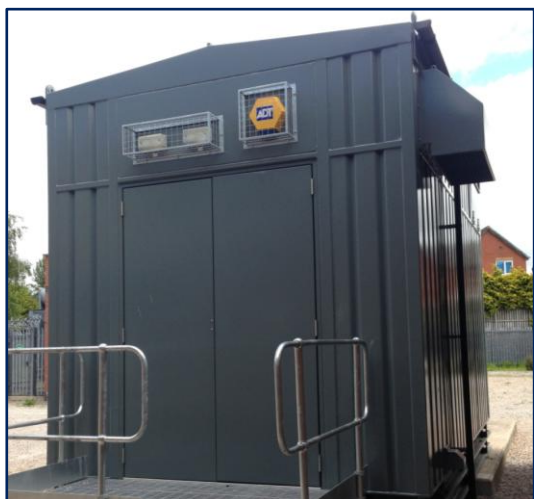
Figure 3.13: I_S -limiter container at Bamber Bridge
