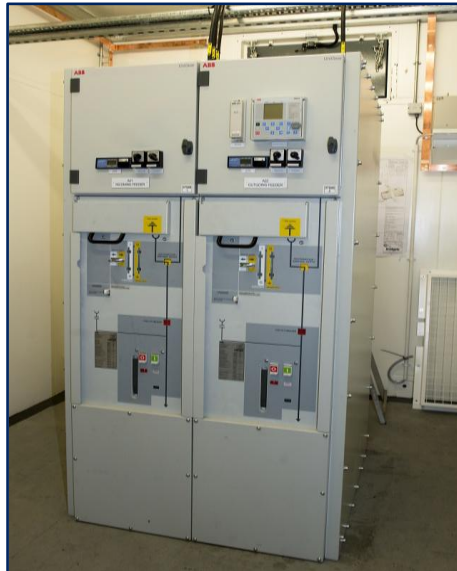
Figure 3.12: Broadheath I_S -limiter bypass CBs
