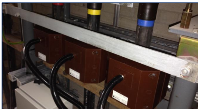
Figure 3.15: I_S sensing unit CTs at Wigan on the Gidlow No1 33kV circuit
