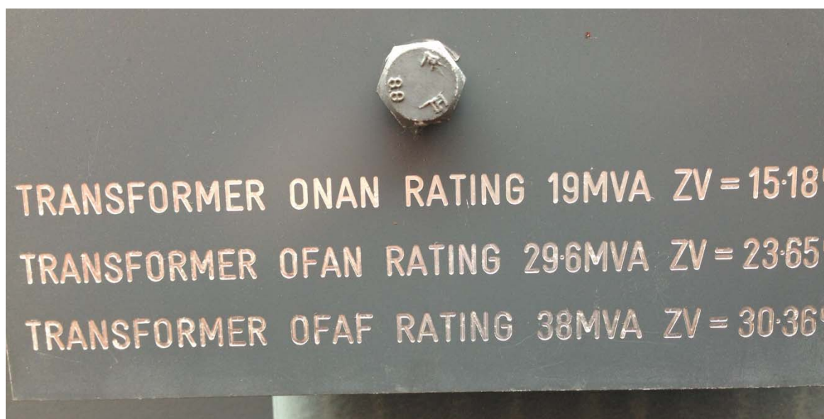
Figure 6-1: Atherton Town Centre transformer nameplate ( Z_{pu} = 0.80 \text{ pu} = 15.18 \times 100 / 19 )
