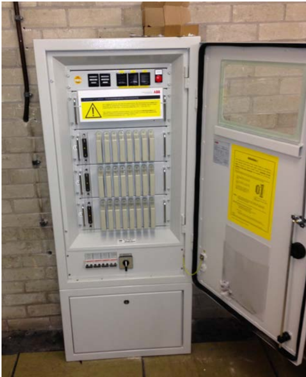
Figure 5d: IS sensing unit CTs at Wigan on the Gidlow No1 33kV Circuit
