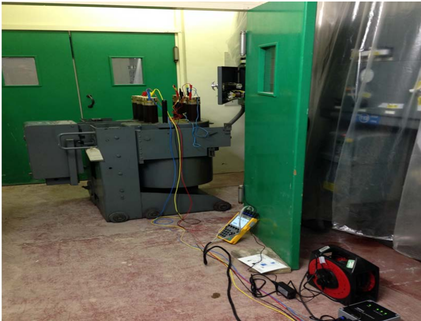
Figure 118: Kelvatek profiler measurement at Denton West
