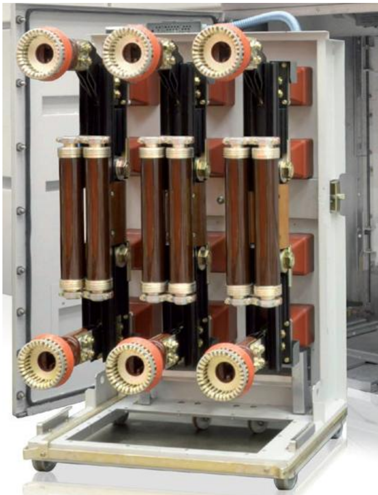
Figure 9.2: View of an Is-limiter truck withdrawn from service (Note that Is-limiter inserts may have only one fuse barrel)
