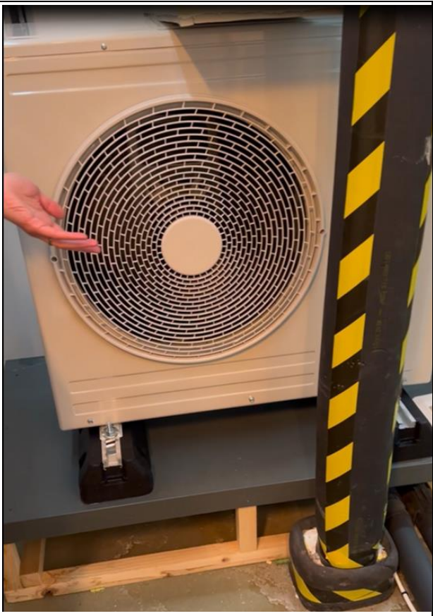
Figure 2—2 Air source heat pump at University of Salford Energy House 1
