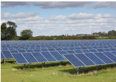
Figure 2-1 - Example ground mounted solar PV system
