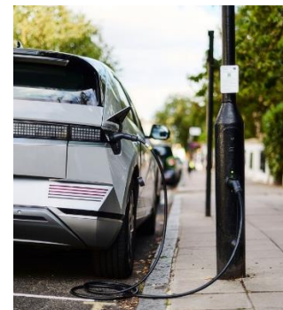
Figure 2-17 Example lamppost retrofit in-street EV charger
