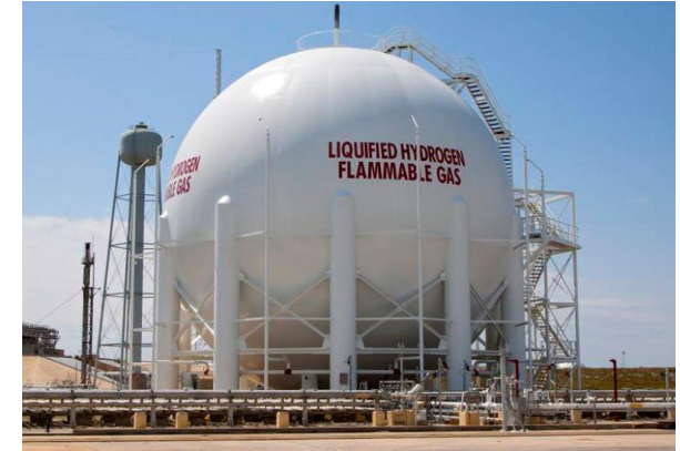
Figure 9: Example of Liquid hydrogen storage vessel [10]
